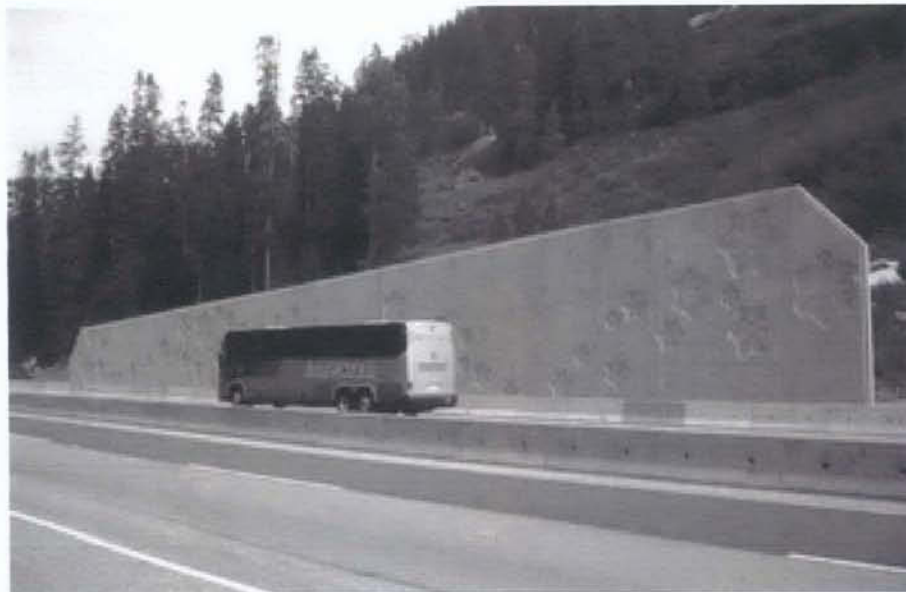
Figure 6. A reinforced concrete wall protecting Highway 5 near Coquihalla Pass in British Columbia. Photographer: British Columbia Ministry of Transportation Snow Avalanche Program.
