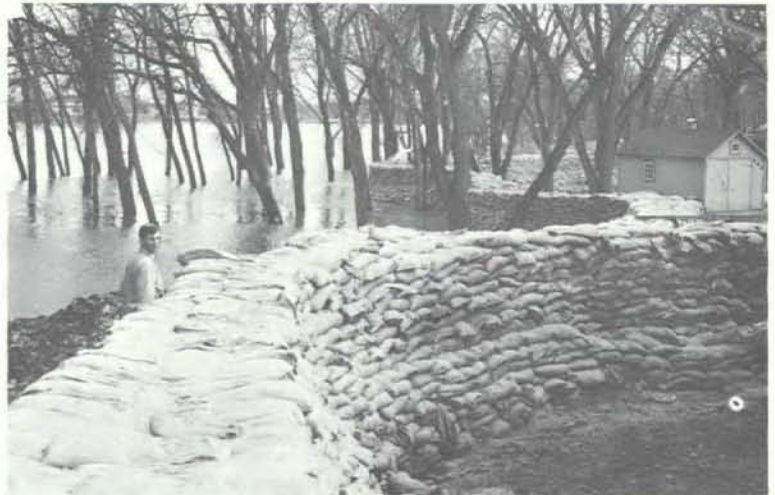
Secondary diking to protect private property in Winnipeg
