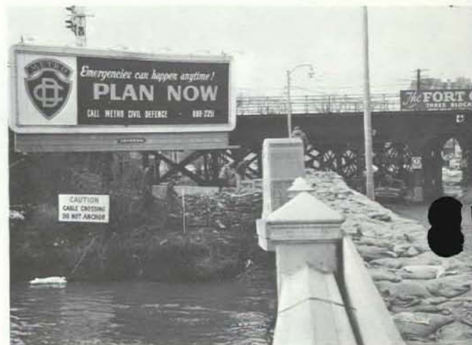
Secondary diking at the Main St. Bridge, Winnipeg
